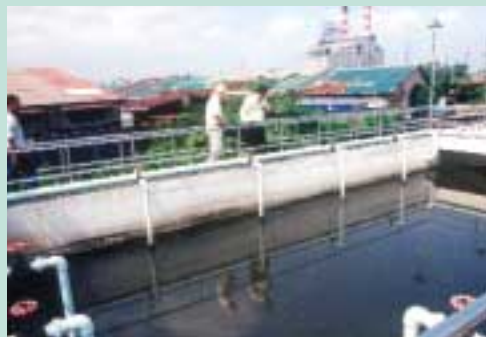
Domestic waste water treatment plant at Unilever Philippines' Manila factory. Treated water from the plant flows through a fish pond before entering a tributary of the Pasig River.
